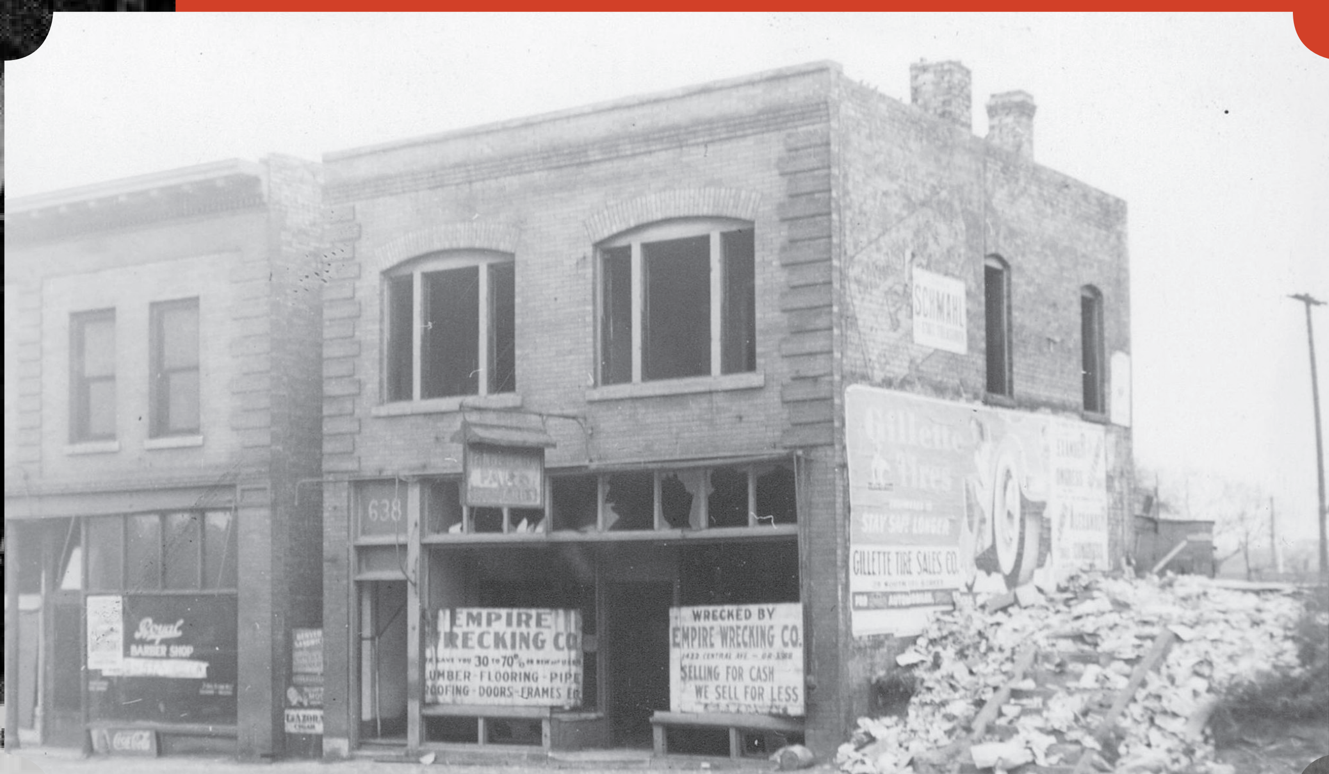
Businesses on the north side of 6th Avenue were demolished between 1936 and 1938. Courtesy Hennepin County Library
