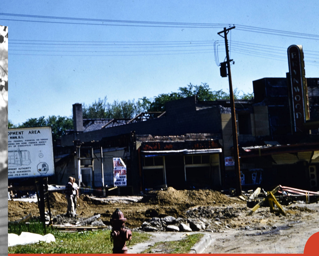
Glenwood Redevelopment Project demolition caused the Homewood Theater to be torn down. The south side of the street was demolished in 1957. Courtesy Hennepin County Library
