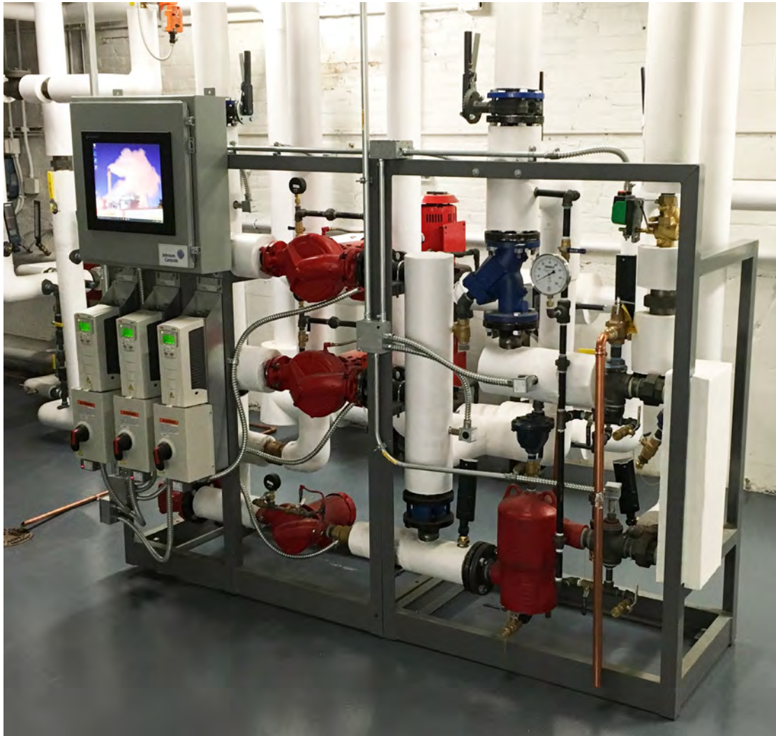
Figure 147: Individual buildings can be designed to easily connect to district energy systems.
