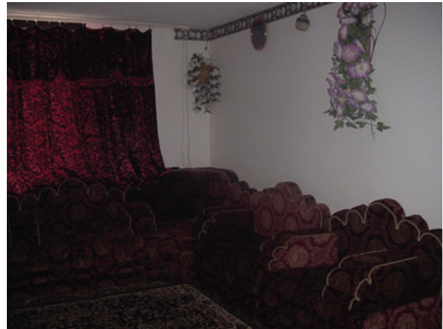
Figure 7 Mould and moisture collect behind these lush curtains.
